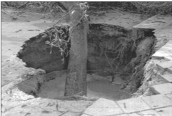
Figure 3. The sink-hole which engulfed part of the Świerczewski Street and a pavement with a tree
